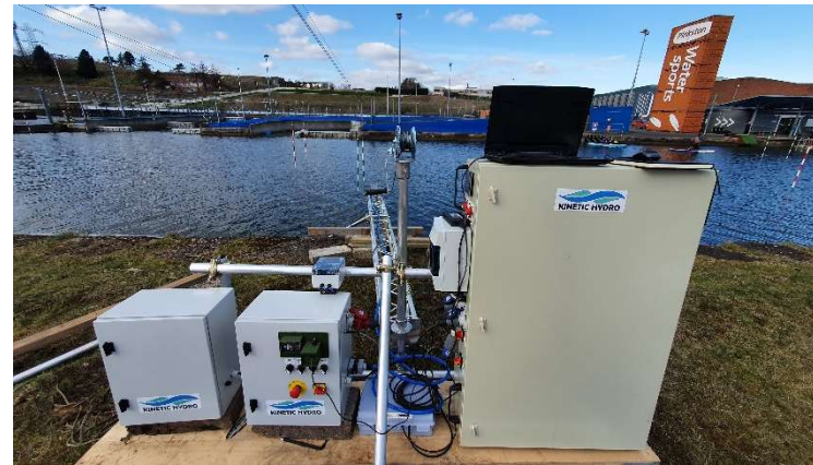
Dump resistors (left), turbine control (center) and mini grid enclosures (right) at our Pinkston Watersports test site in early March.
